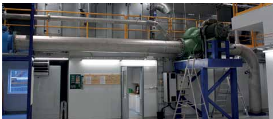
Water flow facility at MIKES-Kajaani, DN500 tube.
